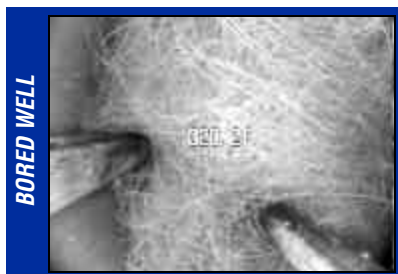
Older wells are more prone to problems such as roots – roots can grow in between the joints of casing. Also, this well's groundwater is under the direct influence of surface water.
