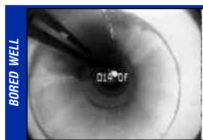
Seepage at the joints of a bored well – shallow water flows into the well carrying contaminants and can pollute drinking water.
