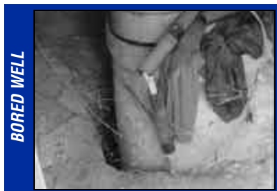
Lack of grouting allows water to seep into the well – water carrying contaminants can pollute drinking water.
