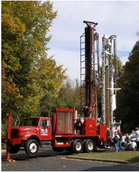
Live drill rigs and drilling equipment, courtesy of several local well drilling companies, were available for up close inspection.
